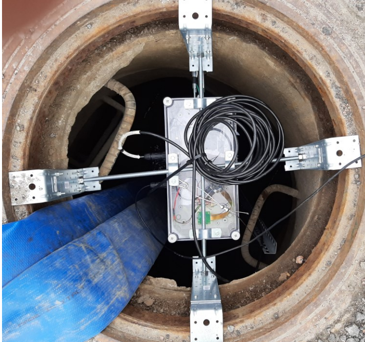
Figure 12: The Turbinator mounted in a stormwater well in Gothenburg. The cable on top of the sensor is a connection to another sensor and is not a part of the Turbinator. Image courtesy of Jens Wilhelmsson, IVL.
