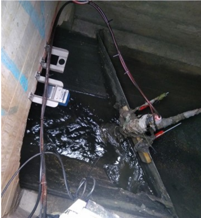
Figure 33: Clogging effect by sensors placed in the water stream, stopping residuals such as paper and plastic. (Image courtesy of Dimitar Kolev, RISE AB)
