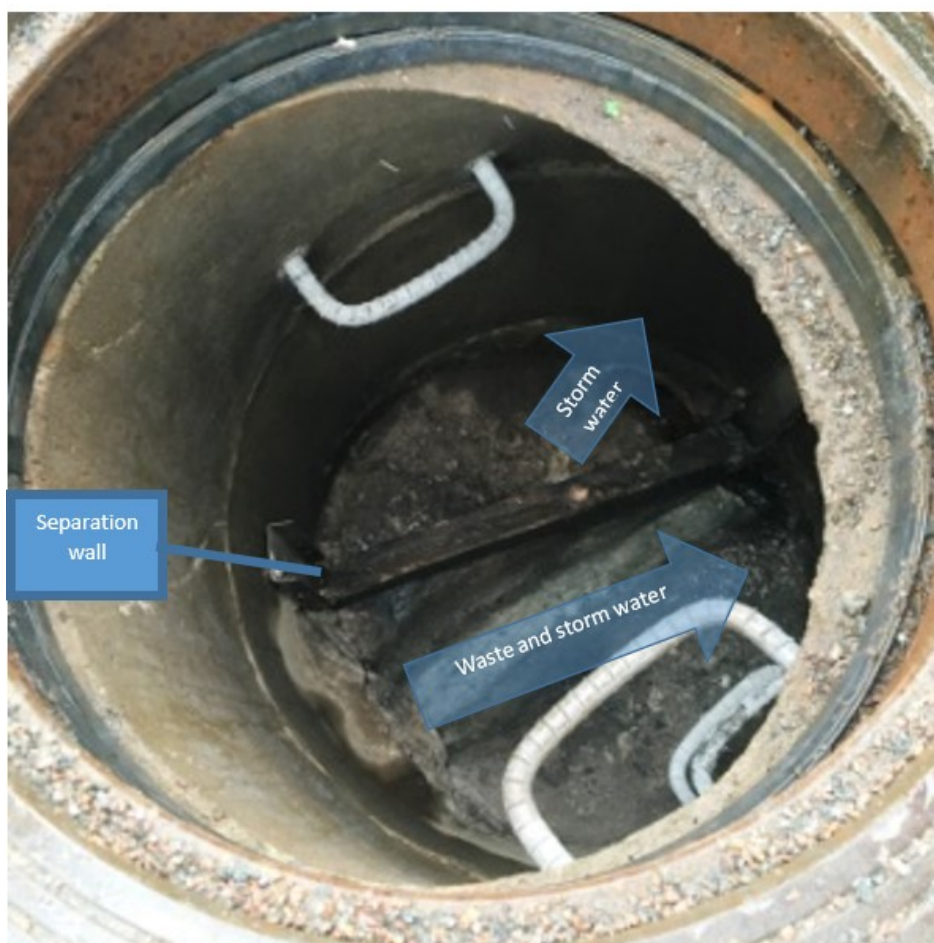
Figure 7: Typical manhole and CSO. Image courtesy of Stefan Lindgren, Talkpool.
