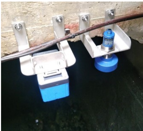
Figure 14: Well at Sävenäs/Renova. Image courtesy of Dimitar Kolev, RISE AB
