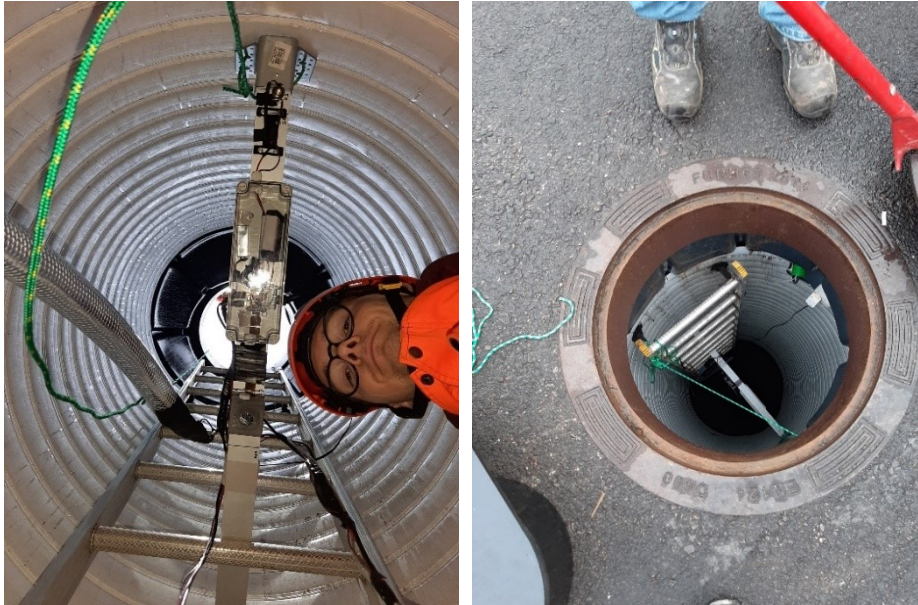
Figure 10: Images from the installation point in Fristad, outside of Uponor's office. Image courtesy of Jens Wilhelmsson, IVL.
